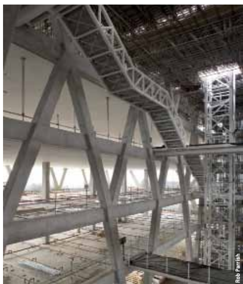
Fasi del cantiere: la copertura a shed e l'atrio Construction site phases: the shed roof and the atrium
